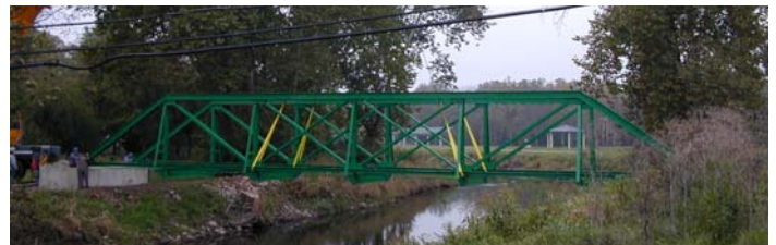
The former Mahalasville Bridge is now painted a vivid John Deere green. White guard rails are being installed.
