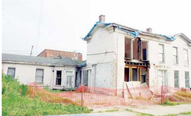
Hite-Finney House (c1855) in June 2004. The city later forced the owners to secure the house and clean up the property.
